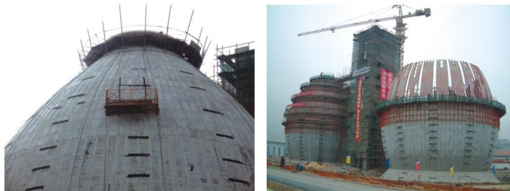
Wuhai Sanjintan Sewage Treatment Plant, China
