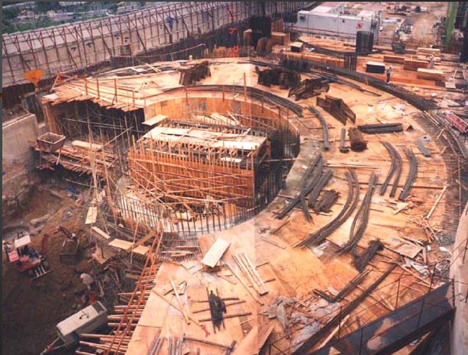
Forming of the vehicular ramp as a means for access for spoil removal purpose during the basement excavation process
