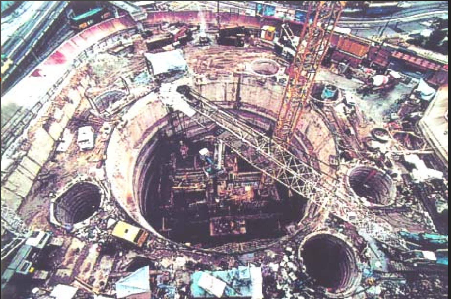
Foundation and core wall work at the same time with the top-down basement
