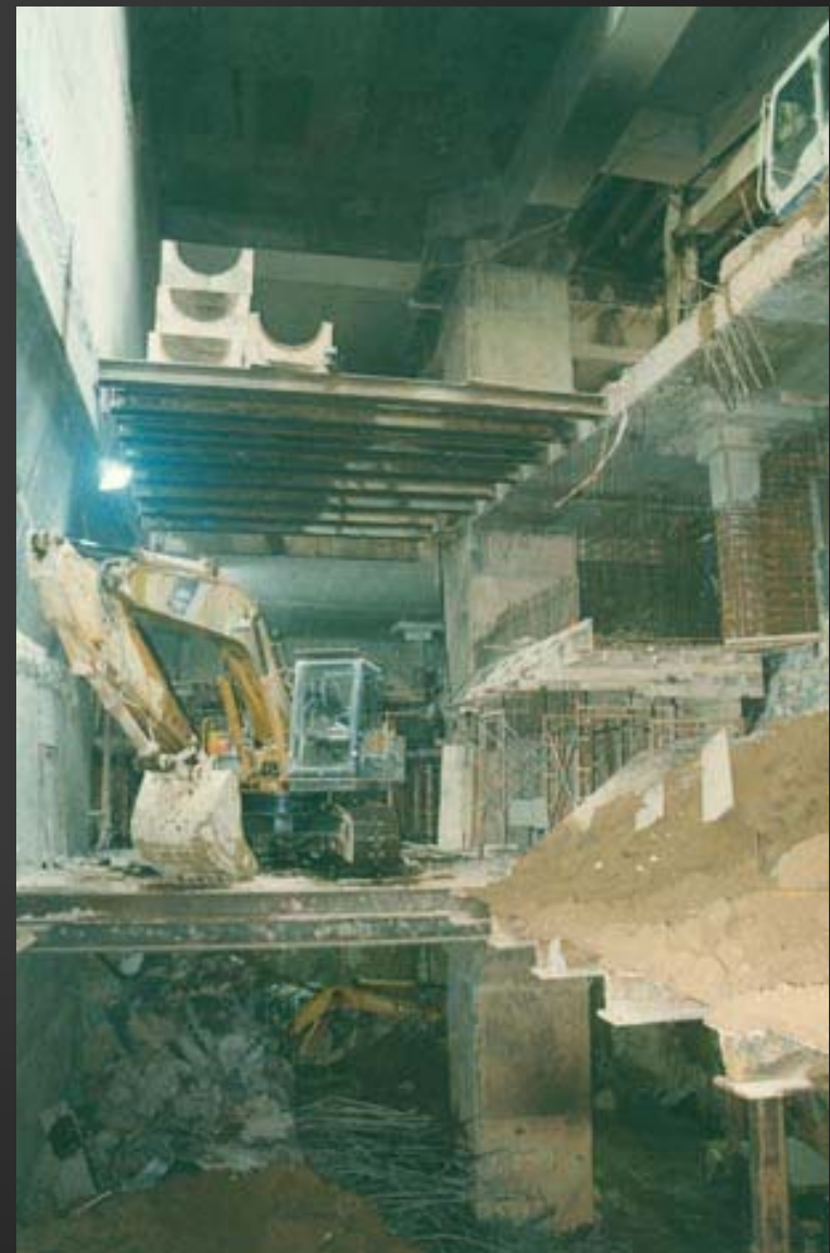
Temporary shoring arrangement to stabilize temporary shaft opening during the basement construction
