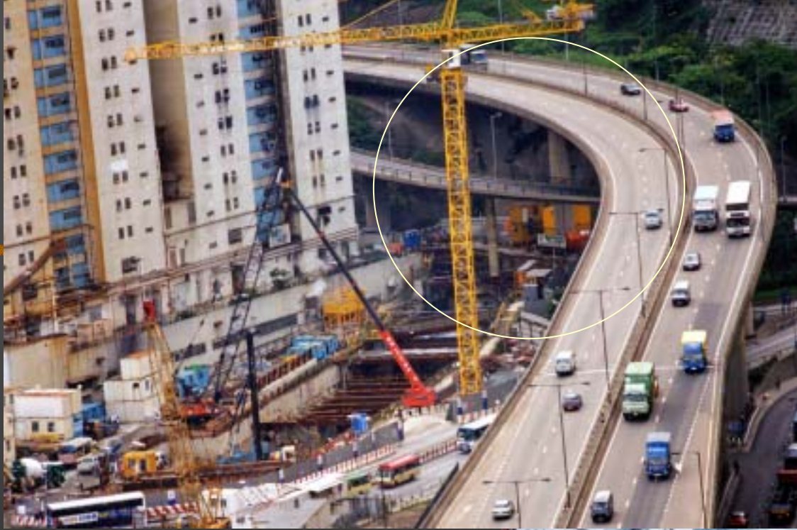
Underpinning to support piers of elevated roadway of Tun Mun Highway at Chai Wan Kok, Tsuen Wan
