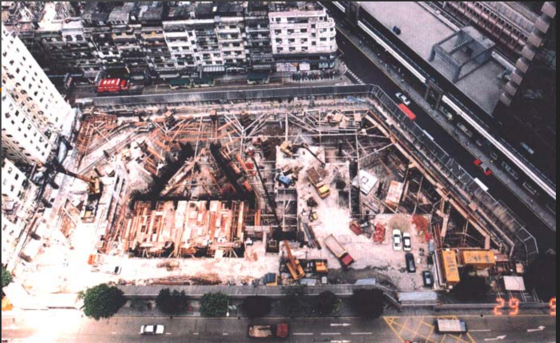
Construction of the new basement slab to replace the old basement structure in phases
