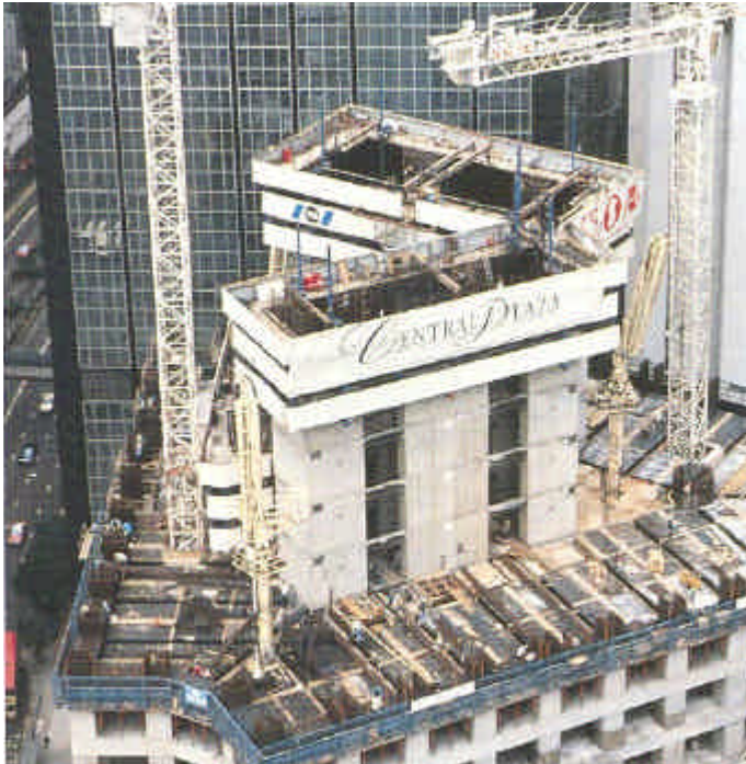
Fig. 2.5: VSL Climbing Formwork is an Efficient Means to Construct Complex Service Cores in High-Rise Buildings
